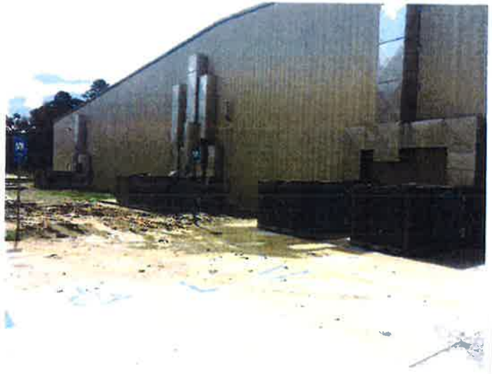
LEFT SIDE GROUND LEVEL CONDENSING UNITS 09/03/2015
