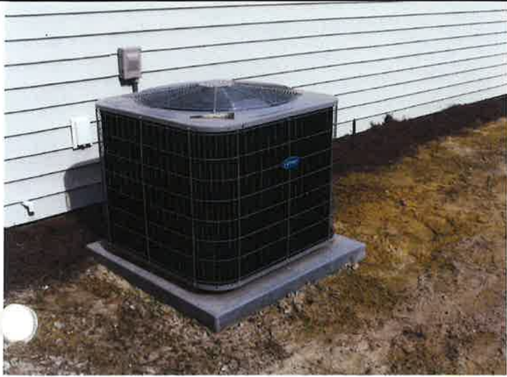
AIR CONDITIONING COMPRESSOR 04/23/2009
